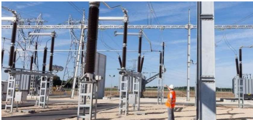
Figure 5-5: Picture of High-Voltage installations inside a 2*25kVca substation
