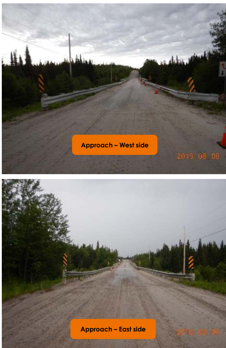
Figure 14 : Wood and galvanized steel Guardrails
