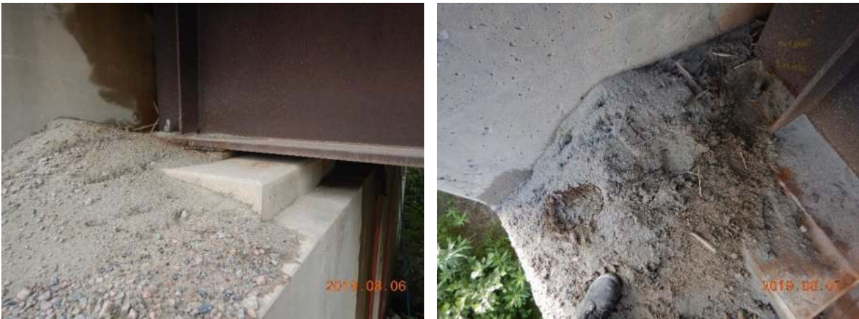
Figure 20 : Debris on the bearing pedestals (West and East)
