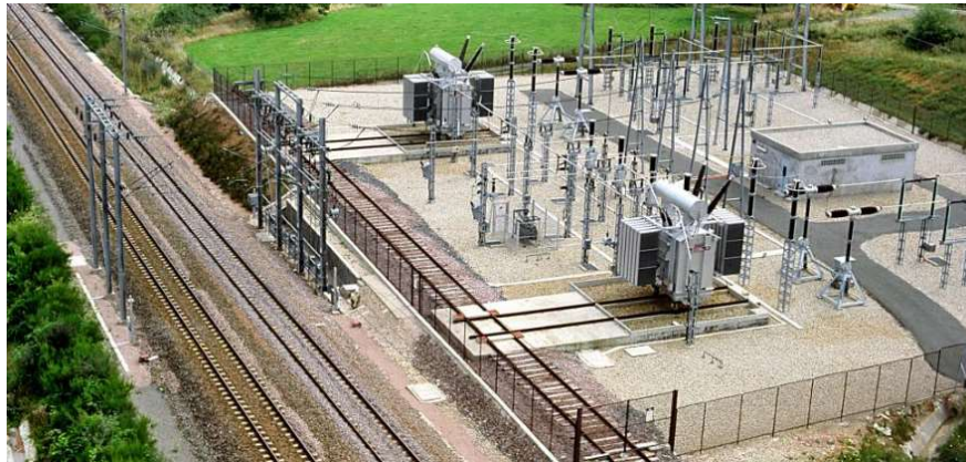
Figure 5-4: Picture of a 2*25kVca substation
