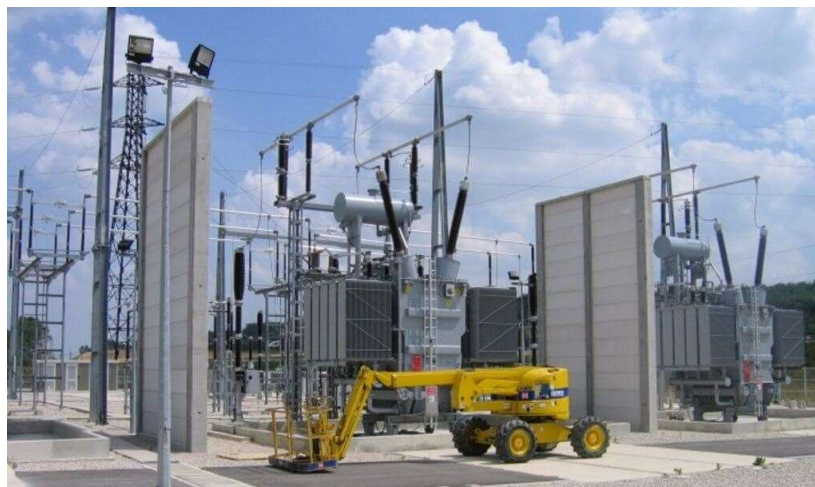
Figure 5-6: Picture of HV/MV Transformers inside a 2*25kVca substation
