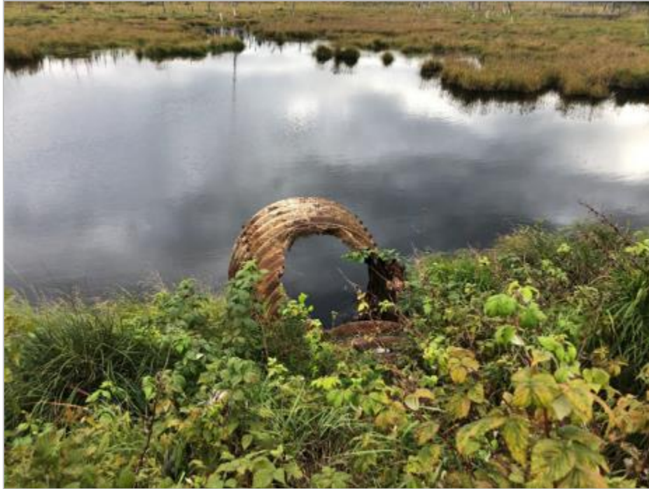
Figure 8.5-101: Existing \pm 1500 mm \varnothing CSP Culvert Crossing Grevet-Chapais Roadbed at KP 220.1 (The culvert is rusted and broken).
