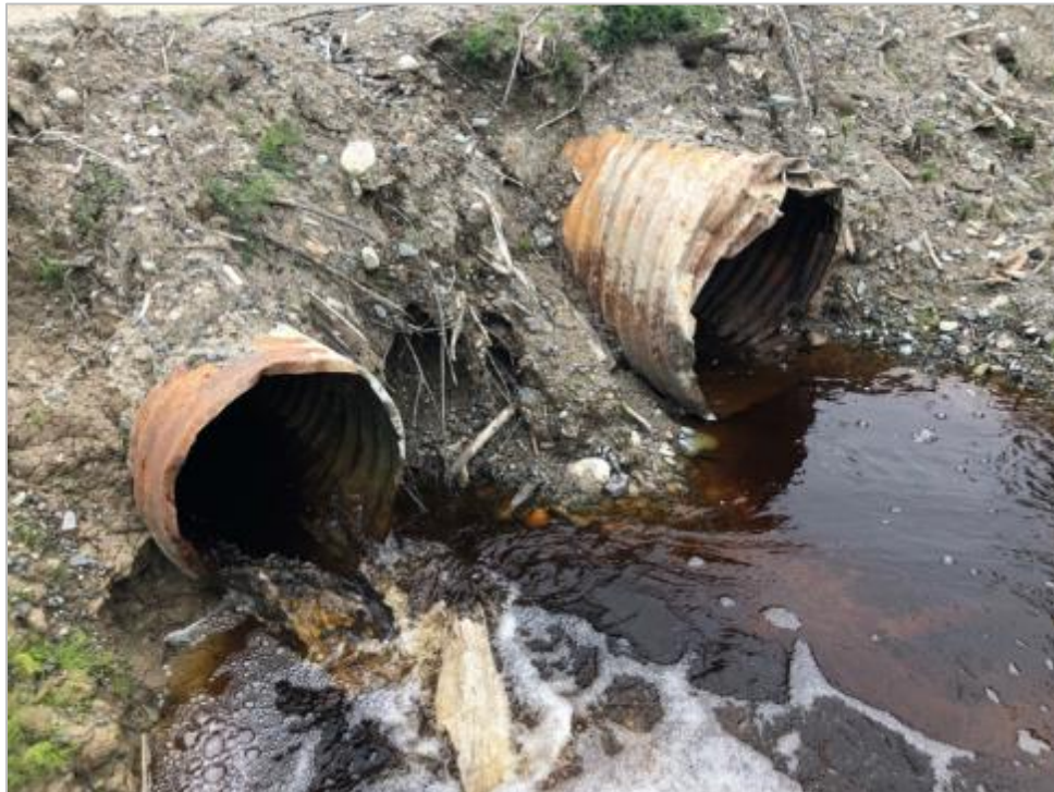
Figure 8.5-100: Existing 1000 mm \varnothing and 600 mm \varnothing CSP Culverts Crossing Grevet-Chapais Roadbed at KP 164.1. (The culverts are rusted and slightly dented but seem functional)
