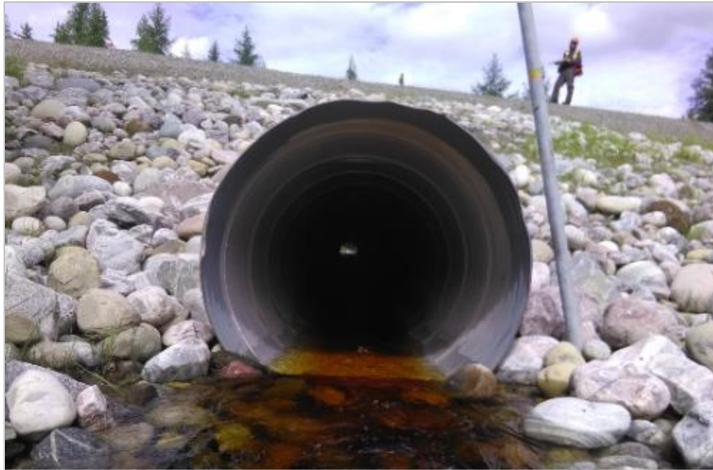
Figure 8.7-10: Site with a lack of crash barrier for a culvert
