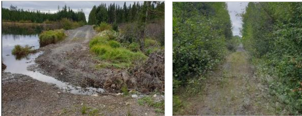
Figure 8.5-34: Examples of Erosion and Forest Encroachment on the Chapais Subdivision Trail
