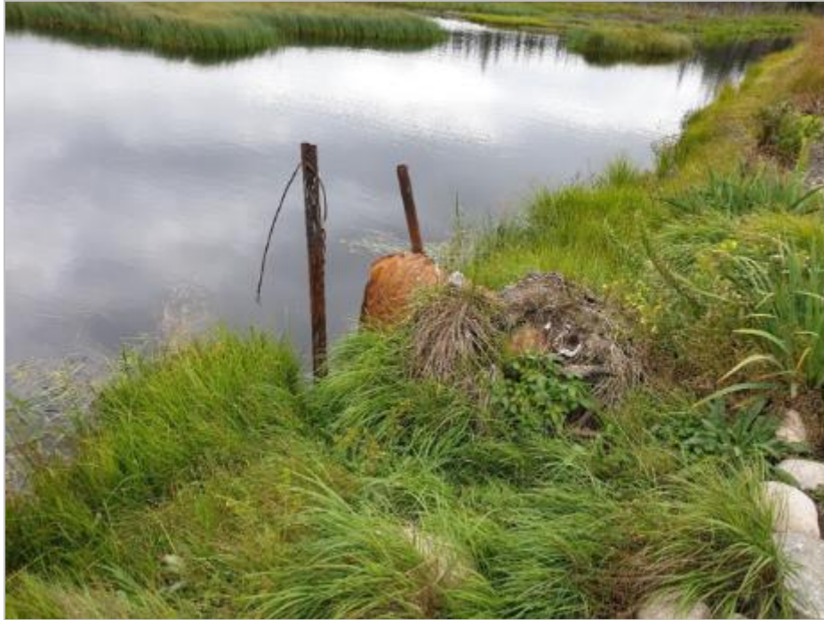
Figure 8.5-99: Existing 600 mm Diameter CSP Culvert Crossing Grevet-Chapais Roadbed at KP 132.0 (The culvert is rusted but seems functional)
